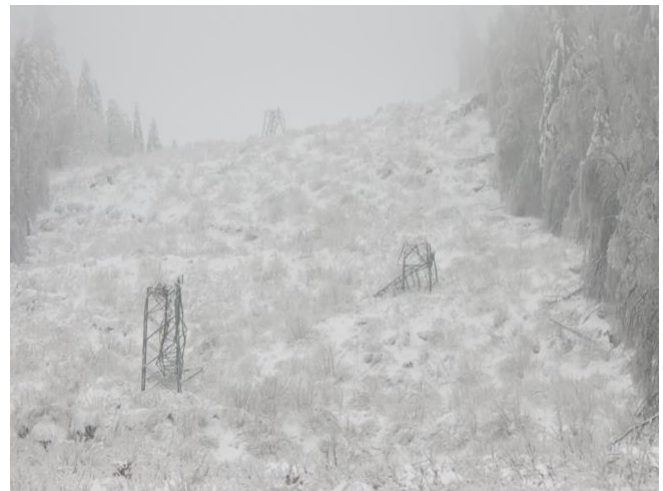
Fig. 4 Disastrous damages on OHL 110 kV Kleče– Logatec [2].
