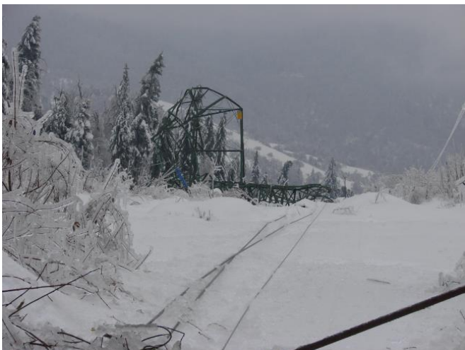
Fig. 3 Disastrous damages on OHL 110 kV Kleče– Logatec [2].
