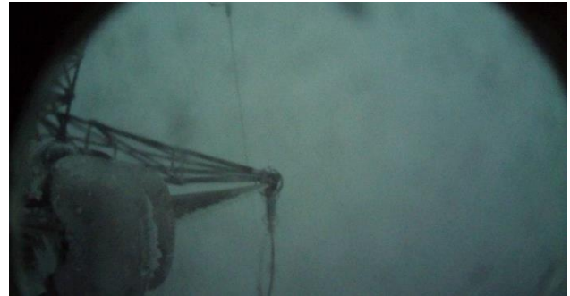
Fig. 13 Real state of a phase conductor.
