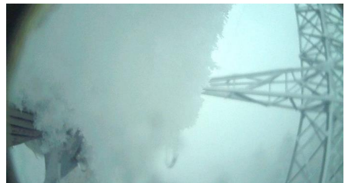
Fig. 15 Real state of a phase conductor.
