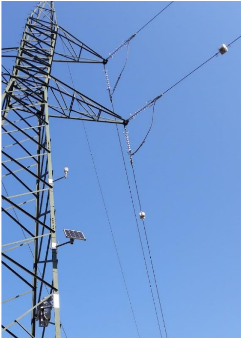
Fig. 11 Tower No 95 (2x OTLM SMART and 1x wether station).
